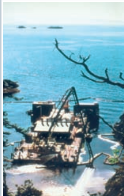
Booms with spray nozzles
