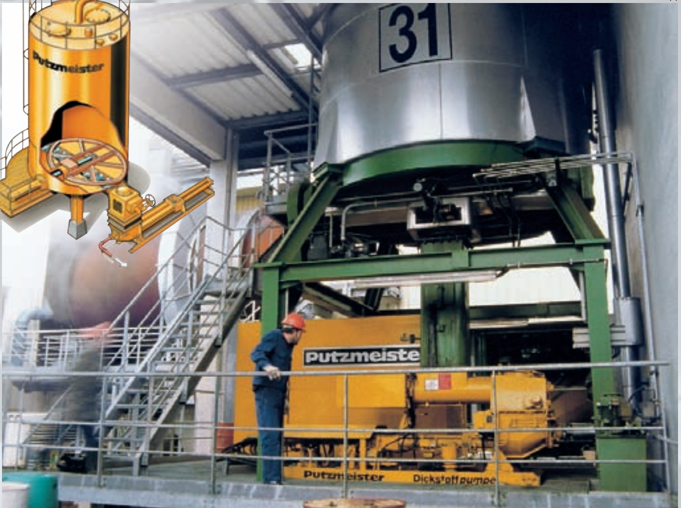
Putzmeister high density solids pump under a silo in a hazardous waste incineration plant (on the top left in systematic diagram)
