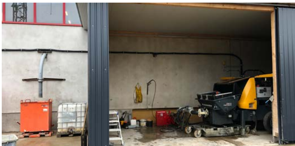
Stationary concrete pump BSA 1408 E in enclosure outside the hall
