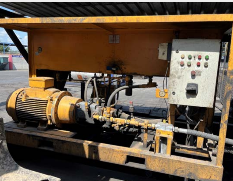
Hydraulic Power unit at Interwaste, Johannesburg
