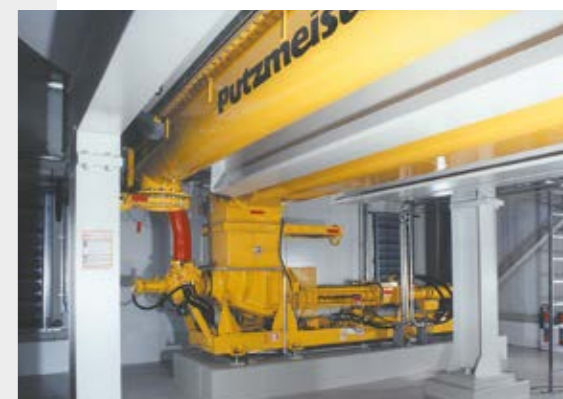
Solids handling pump KOS 1460 and emergency discharge auger beneath a 500 m 3 storage silo
