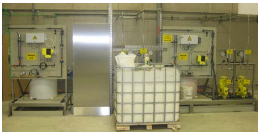
BLI preparation and dosing station incl. control cabinet
