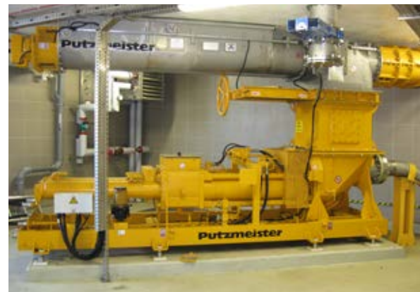
Twin feeding screw SHS 2442 SH delivers the sludge out of the concrete silo into a KOS 1080 piston pump with service gate valve
