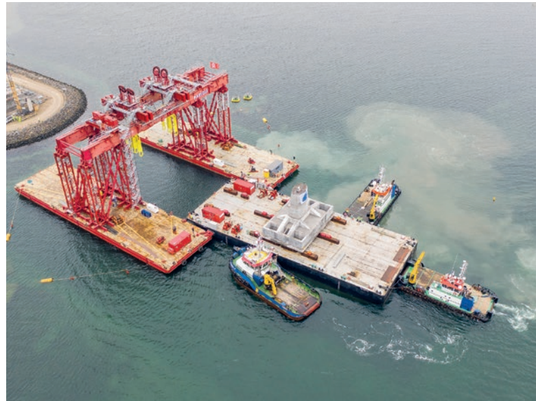
Fig. 8: The first prefabricated foundation with two pillar segments is transported to the assembly site and installed with a crane catamaran (copyright: Vejdirektoratet)
