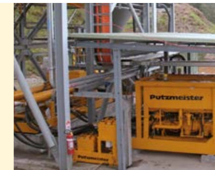
HSP 25100 HPS, PCF-Ventile, Hydraulikaggregat HA 400 + 400 E-SP
