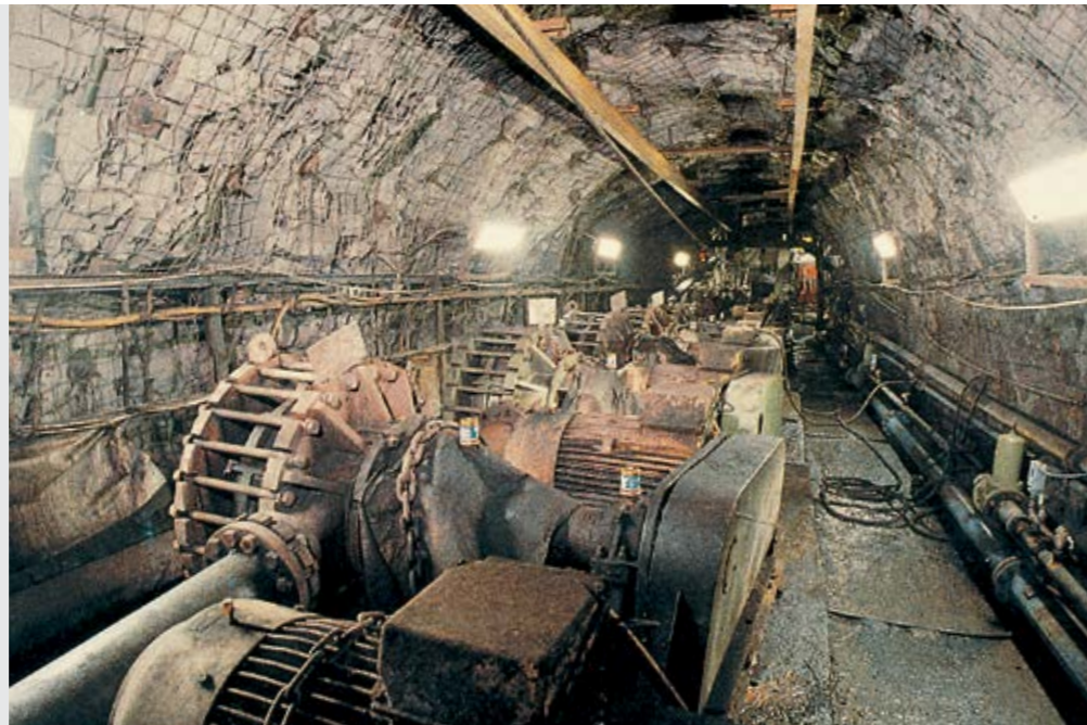
View into the former sludge pump room on the 686-m level invert. The 12 single chamber centrifugal pumps are connected in series and convey the sandy water over 141 m to the next 545-m level invert.
