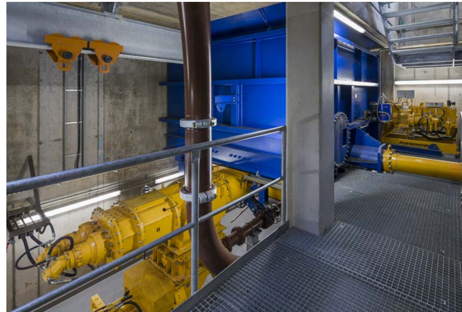
A crane device is fitted over the pump
