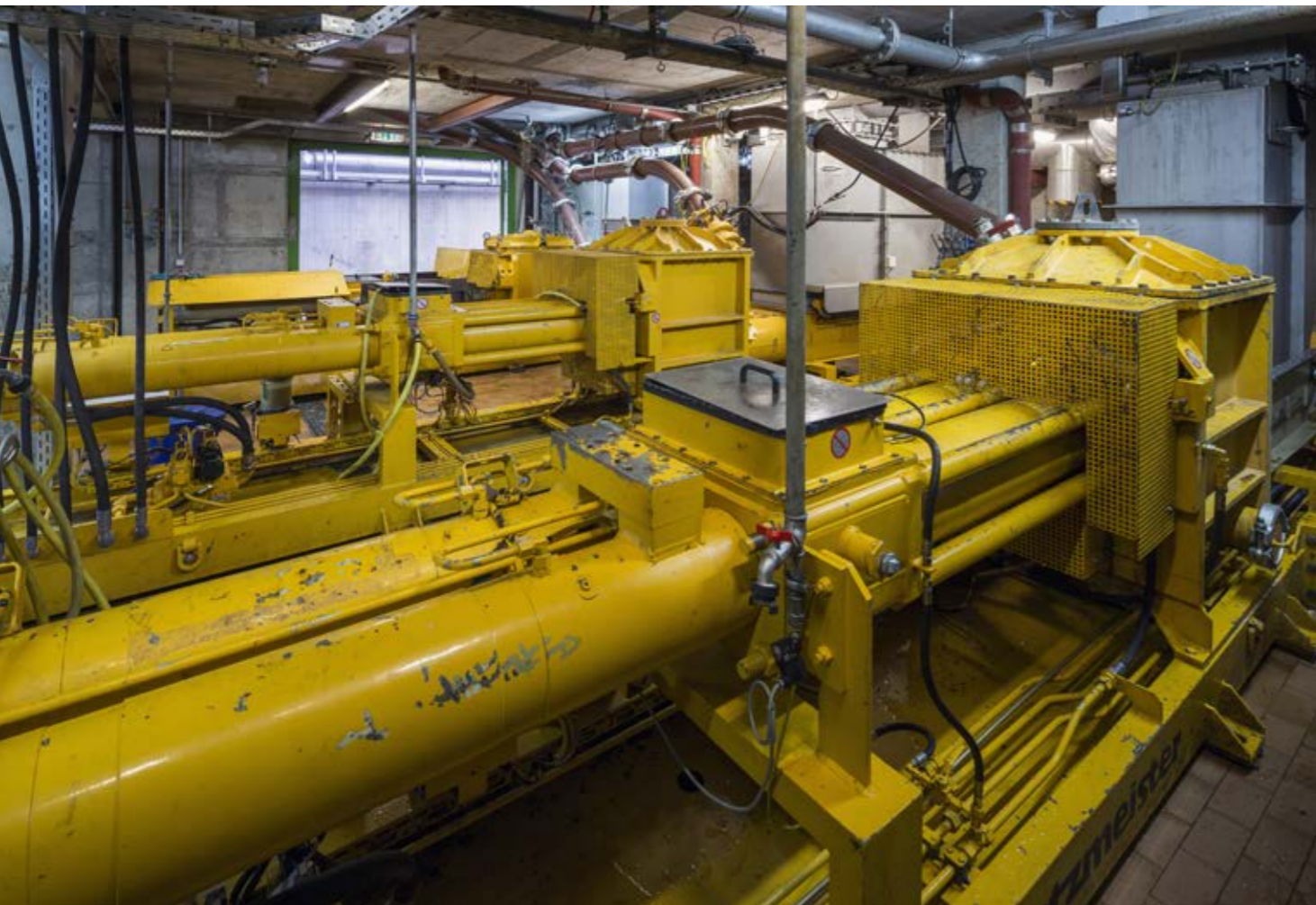
The hot sludge department: Two KOS 1070 HP LIB and one KOS 1040 HP LIB under the three dryers convey the 65 to 70 °C hot sewage sludge
