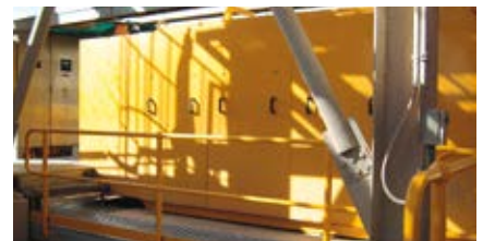
Hydraulic unit with control cabinet
