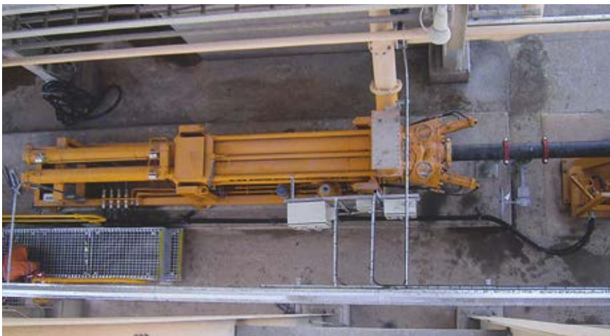
General overhead view of pump with emergency drain valve between pump and power damper
