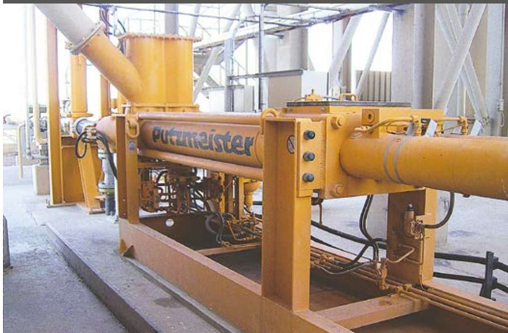
Pump with intake shaft
