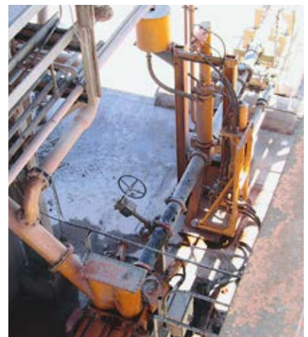
Power damper with delivery line
